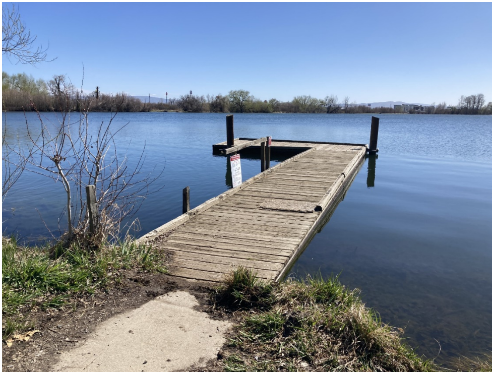
Photo 1. Existing boarding float with missing planks and broken boards
